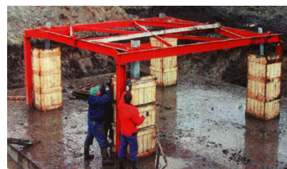
The foundation for a lattice tower takes approximately four weeks to produce.
